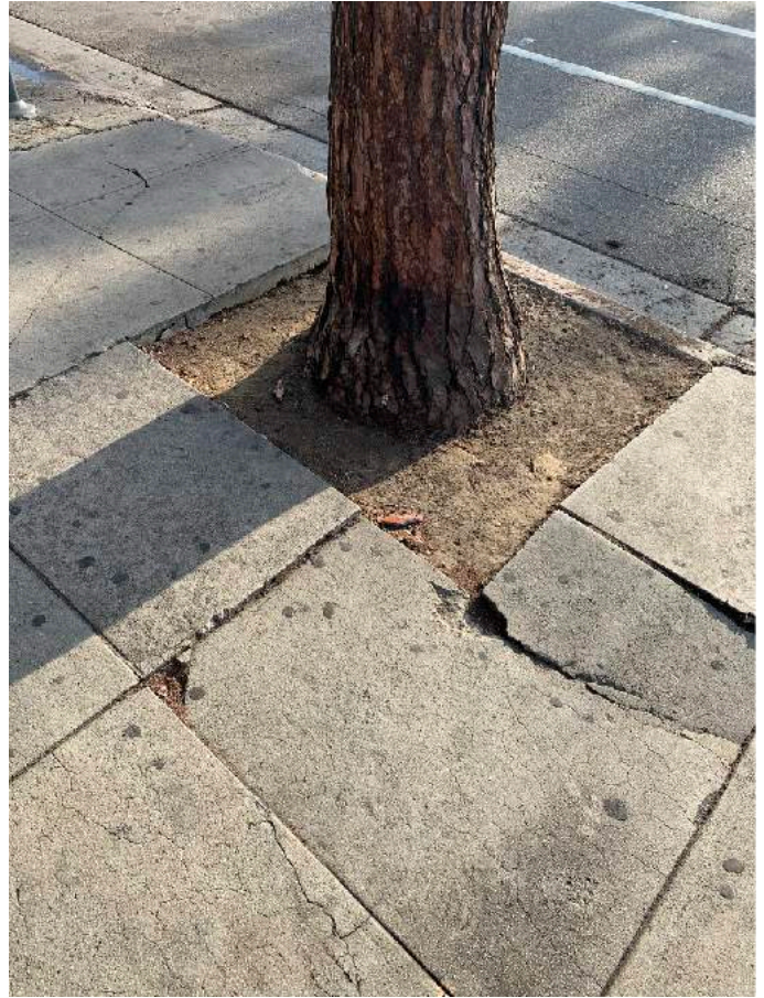
PHOTO 7 -Note hardscape around Canary Pine #6 is lifting
