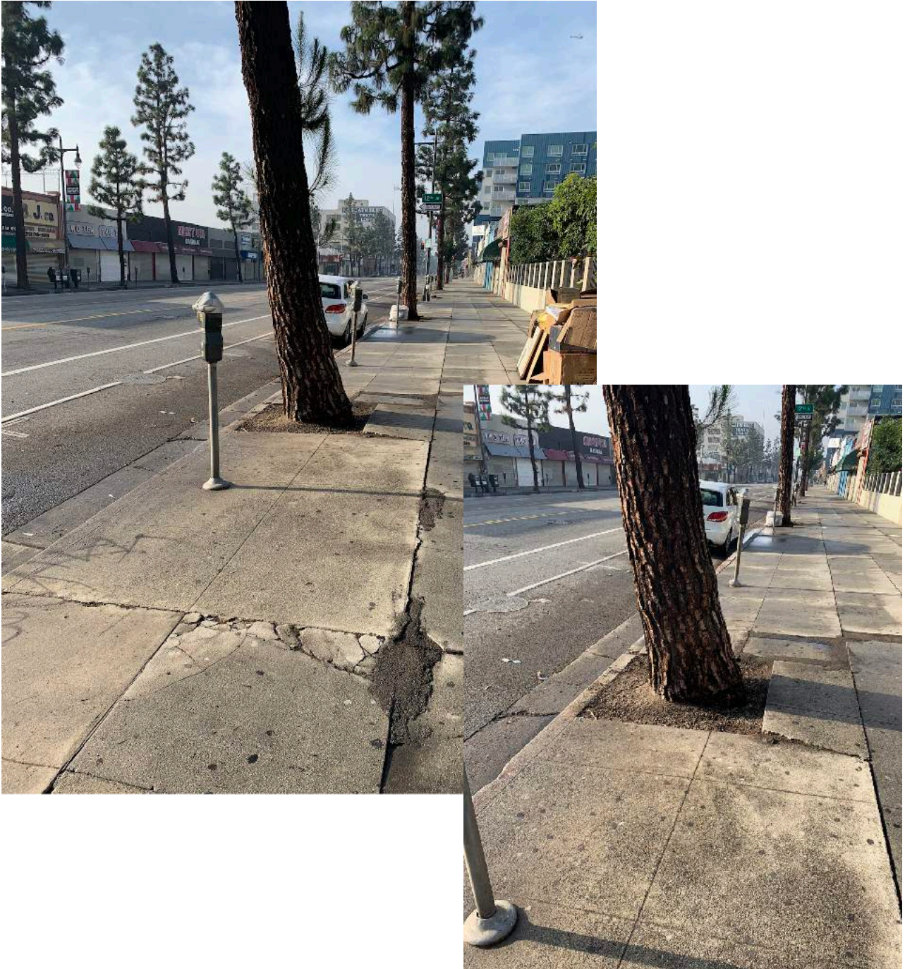
PHOTO 2 - Canary Pine #3 - hardscape lifting around tree base. This tree is recommend for removal and replacement.
